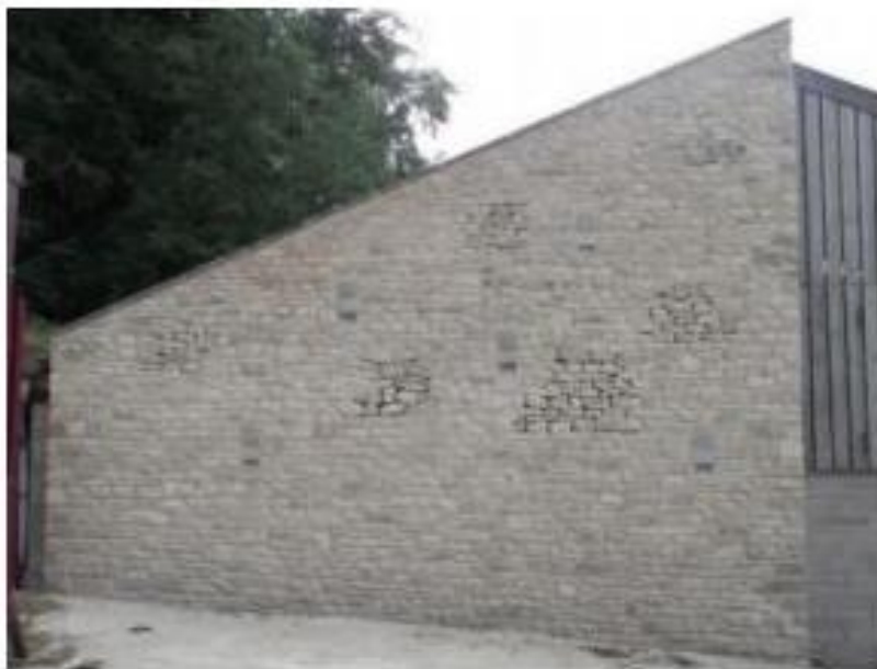
Figure 3. New purpose-designed Bat Wall constructed on the east-facing gable wall of an existing hay barn; includes multiple crevices between the stonework leading to internal cavities and five wall integrated IFR Schwegler Bat boxes.
