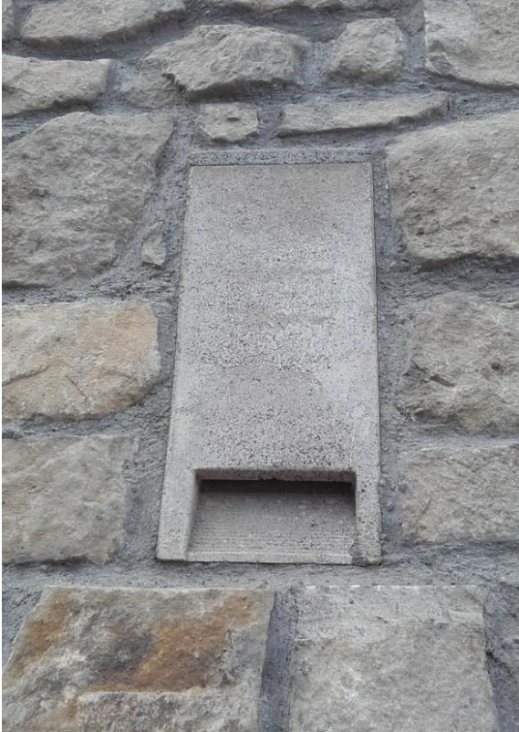
Figure C: Bat tube inserted into external parapet walls of Ross Bridge, Co. Clare.
