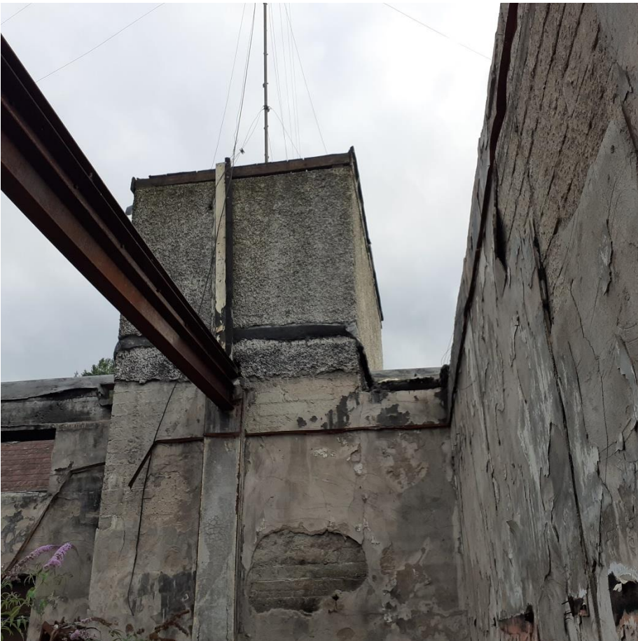
Plate 2a, b: Derelict golf club house.
